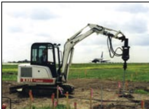
Airport weather station
